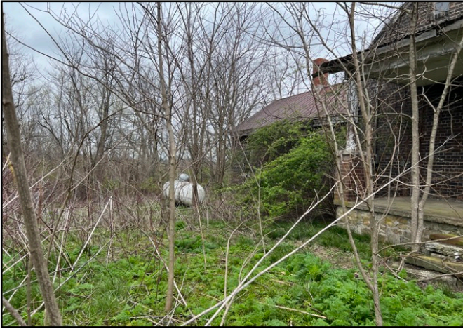
13. View of butane gas tank, on the western side of the house.
