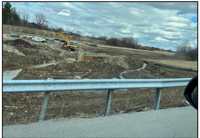
12. Example view of earthwork northwest of the site at the intersection of Caleast Road and Duncannon Lane.
