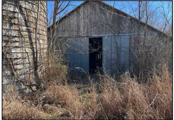
8. View of barn #2 adjacent from barn #1. Also showing silo next to the barn, facing east.
