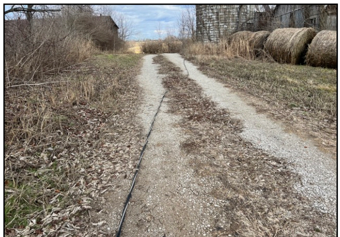
24. Example of "downed" power line near the barns, facing north. - Note - Line was not live.
