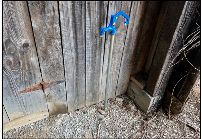
8. Example of fresh water pump inside barn #3.
