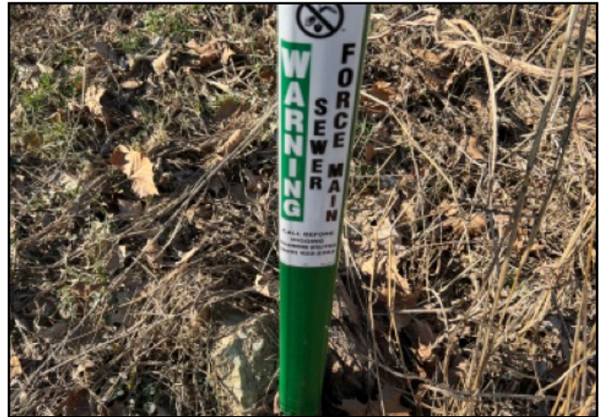
22. Example of 12" PVC sewer line that runs diagonal through the center of the southeastern quadrant.
