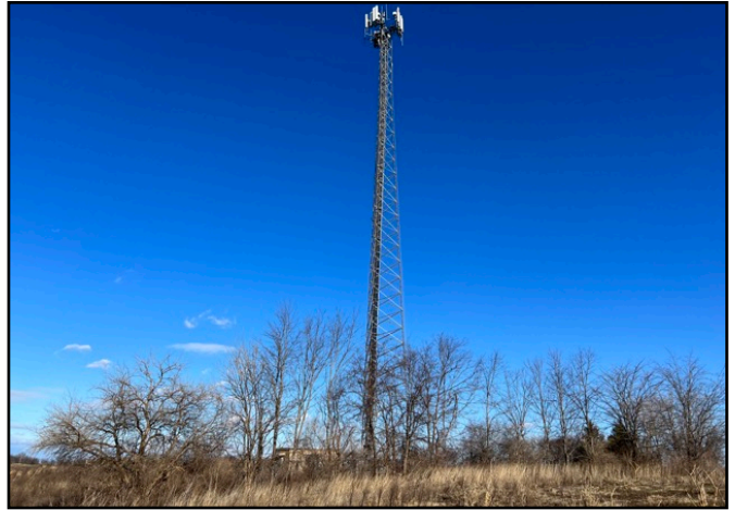
2. View of cellular tower from uppermost quadrant. Facing northeast.
