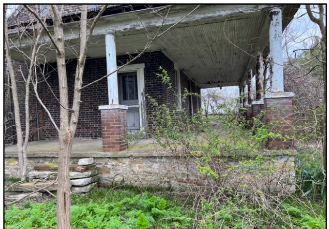
12. Example of abandoned house, facing east.
